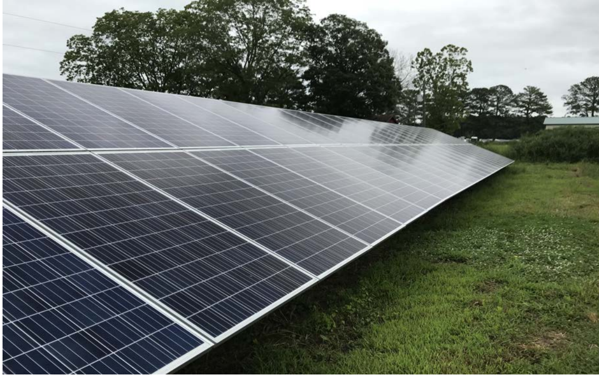
Great Bay Solar Project (118 MW) Westover, Maryland
